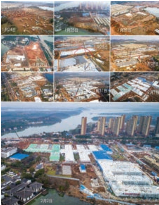
Fig. 10 | Building site stages of the Huoshenshan Hospital in Wuhan, built in 10 days (source: mfa.gov.cn).
