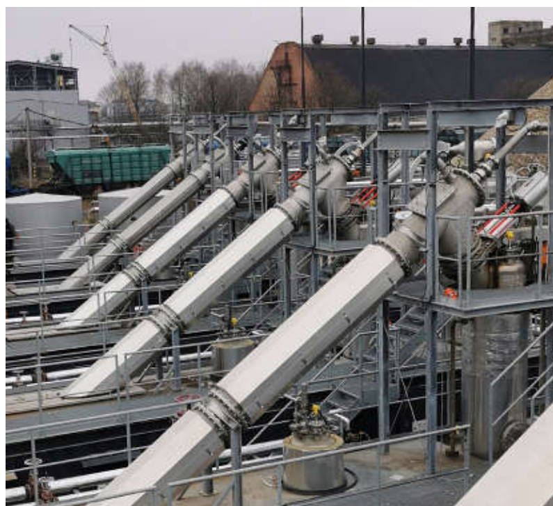
Figure 6.9. SE of the Teofipol plant in Ukraine
