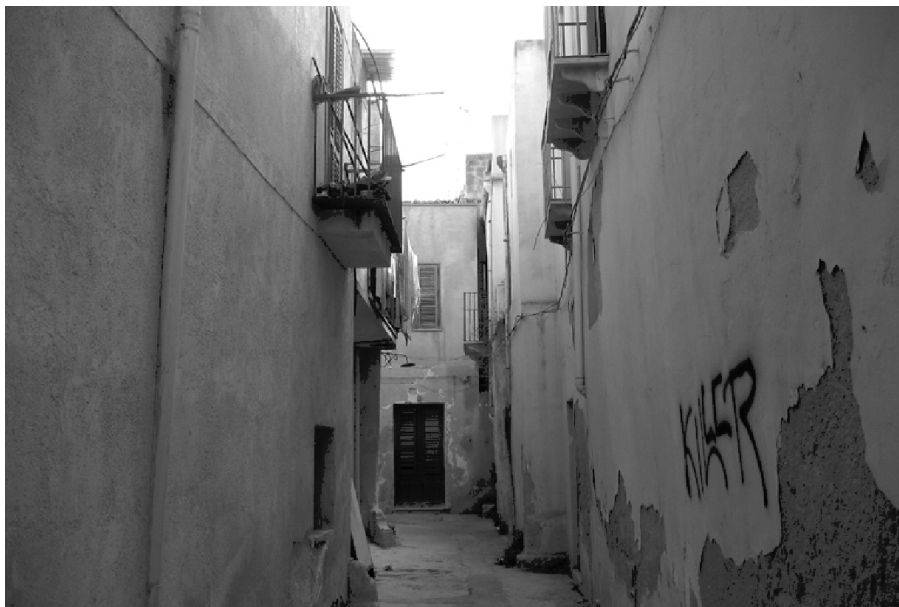
Fig. 2 The deterioration of the part of the historic centre that is inhabited by the Maghrebian community (Photo by Vinci I)
