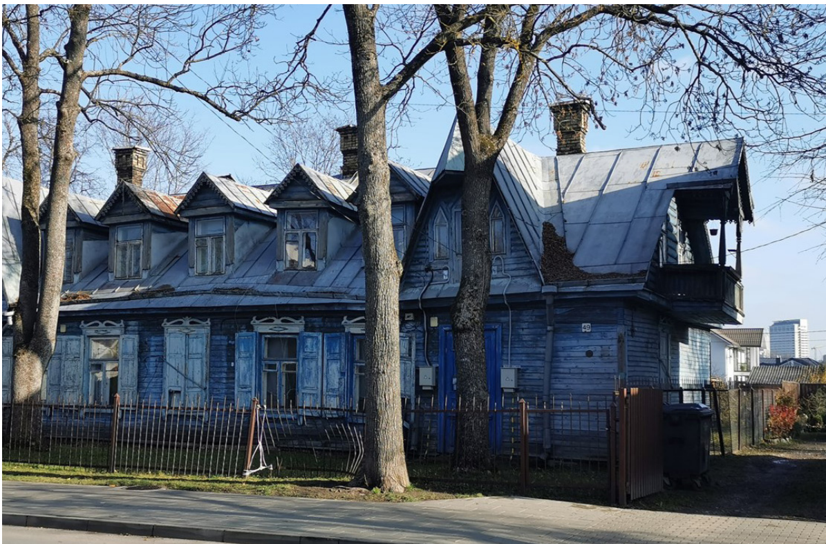
Fig. 5. Example of wooden architecture in Lithuania, object of a necessary rehabilitation intervention (photo by the author).
