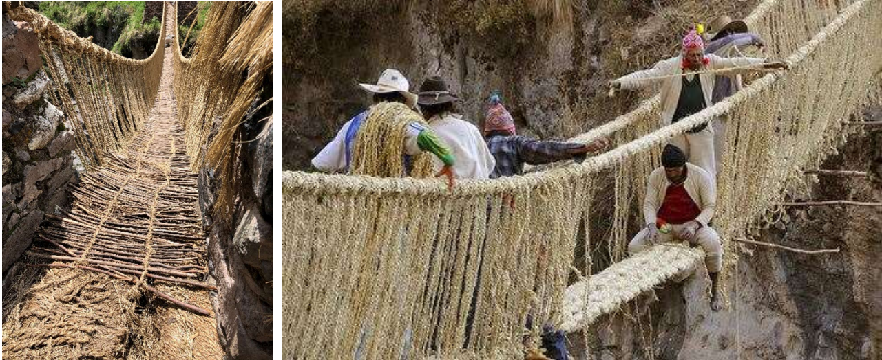
Fig. 4: On the left, the walkway of the bridge. Right, a moment of the reconstruction.
