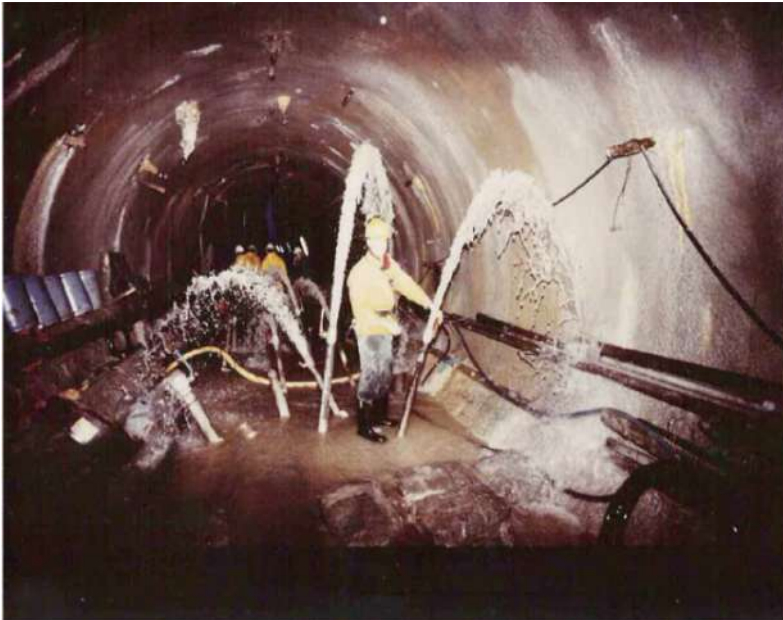
Fig. 4.10. Water inflows during LEP tunnel construction.
