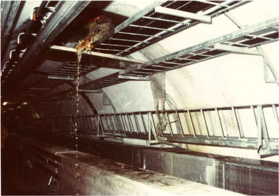
Fig. 4.11. Failure of tunnel concrete lining in 1990.
