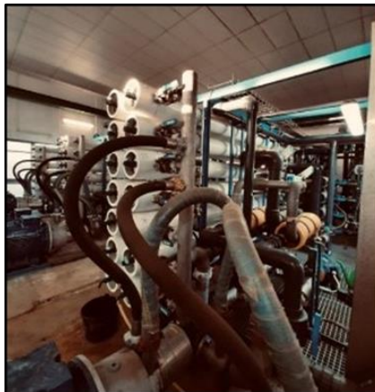
Figure 2: Sataria SWRO Plant, Pantelleria (Italy).
