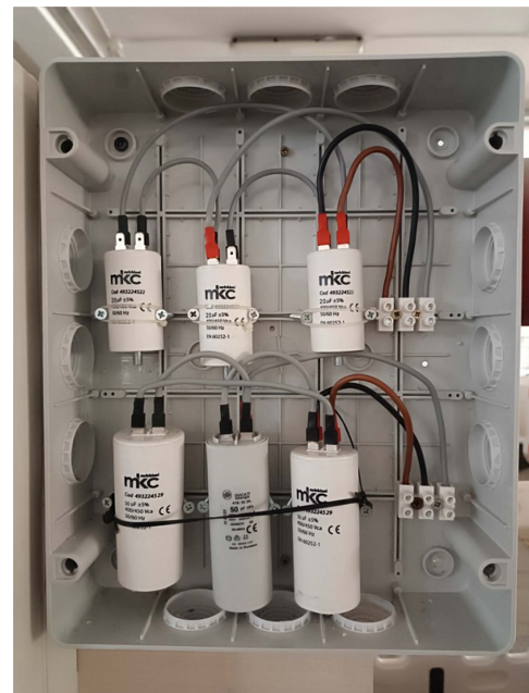
FIGURE 3. Photo of the capacitor bank used for the SEIG excitation.
