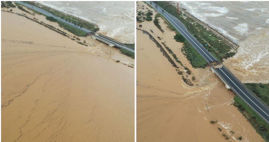
Figure 6. Barrier breaching at La Playa beach and collapse of SS 195 during the compound sea and lagoon flood of 10 October 2018.
