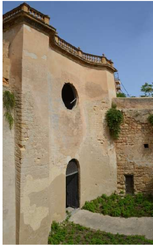
Figure 3. View of the main façade of the church of “Santa Maria della Grotta”.
