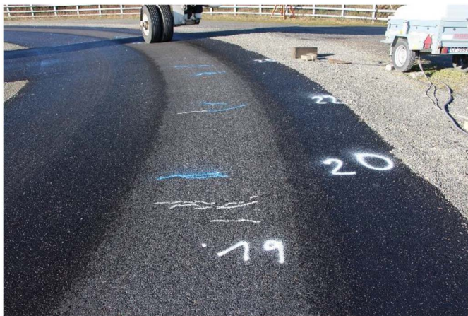
Fig. 12. Condition of the pavement after 1.0 million load repetitions.
