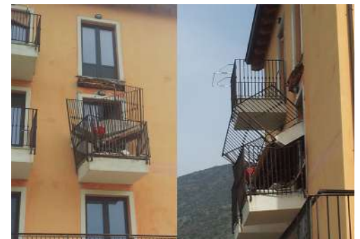
Fig. 2 – Some photographs concerning the conservation status of some buildings of the C.A.S.E. Plan in L'Aquila
