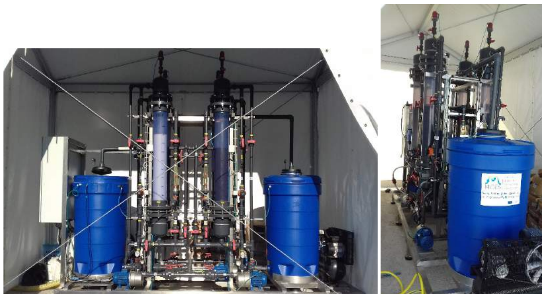
Fig. 1. Novel media filtration pilot plant.
