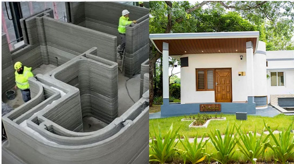
Fig. 10. Tvasta's first structure is a single-storey house, a 600-sq ft unit, created in collaboration with Habitat for Humanity's Terwilliger Center for Innovation in Shelter at the IIT-Madras campus.
