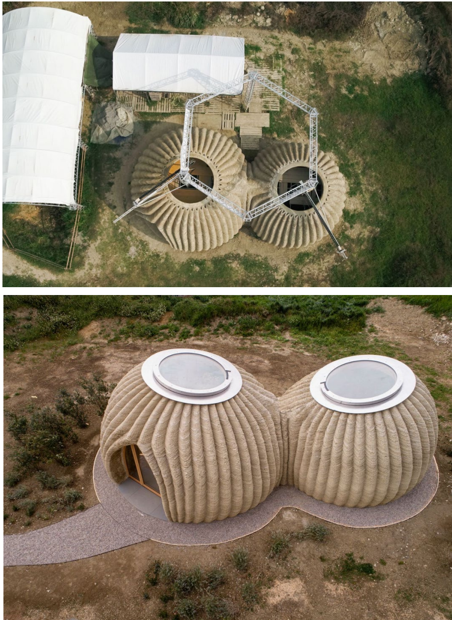
Figs. 8. 9. TECLA by Mario Cucinella in collaboration with WASP. View of On-site 3D printing in Massa Lombarda, province of Ravenna, Italy
