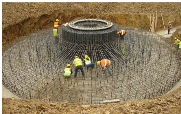
Fig. 1 Steel reinforcements in shallow foundations for wind tower (photo by the author)
