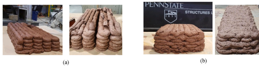
Fig. 12. Freshly printed and cured 3DP beam using cob mixture (a) Before modifying mixture for shrinkage and (b) after modifying mixture for shrinkage [25].
