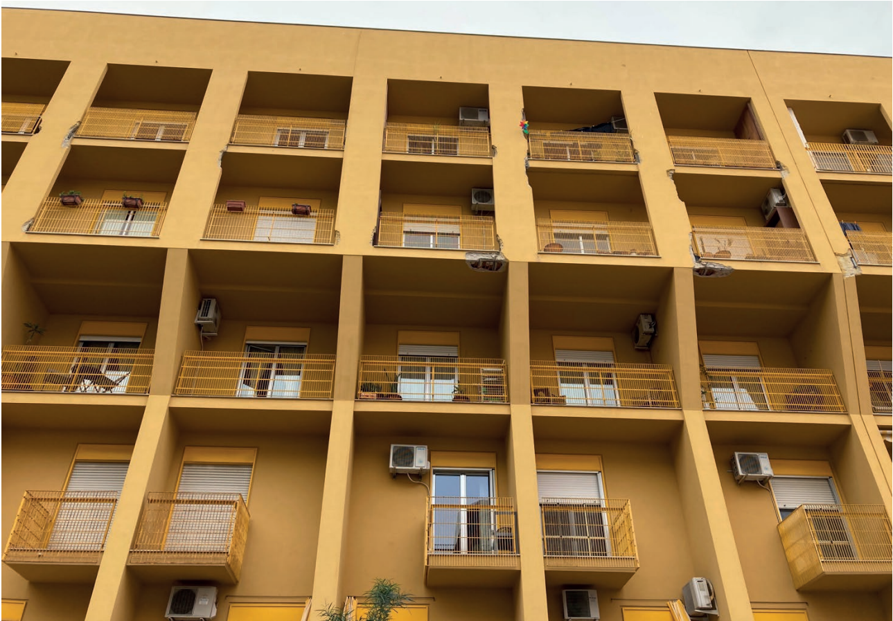
Figure 9 | Palazzo Giallo in Cefalù (PA), designed by architects Culotta and Leone and built in the early 1970s. The facade, after about ten years after the maintenance intervention, shows again signs of degradation (Ph. M.L.G. 2022).
