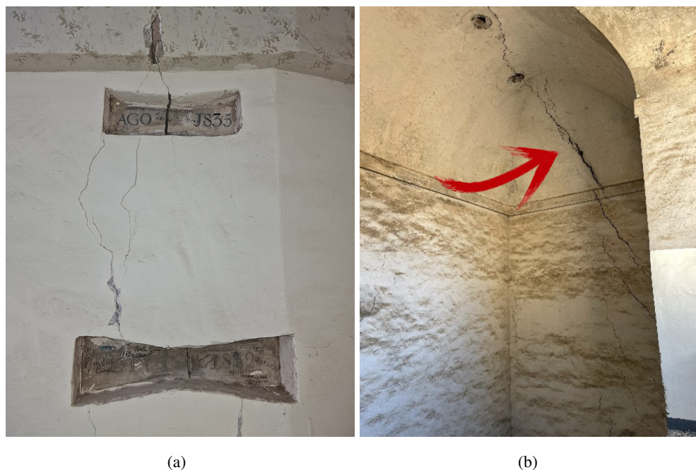
Figure IV.13: Crack pattern at the level of the second corridor: (a) ancient marble tell-tales inside the corridor; (b) diagonal fractures across the vaults at the Catafalchi-Burbera level.
