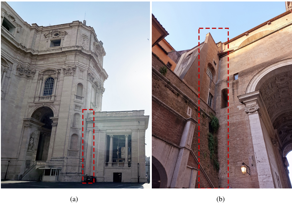
Figure IV.5: South and north towers of St. Peter's Basilica: (a) detail of south tower-Bernini's outer colonnade connection; (b) detail north tower-adjacent buildings connection.
