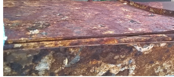
Particular 2. Presence of rust
