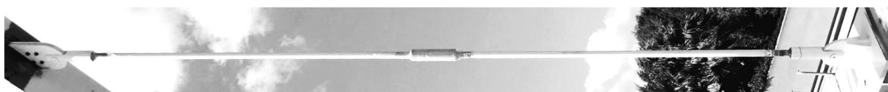
Figure 5. View of the whole hanger with the top (at the left side) and bottom (at the right side) connections with the central tensioner.
