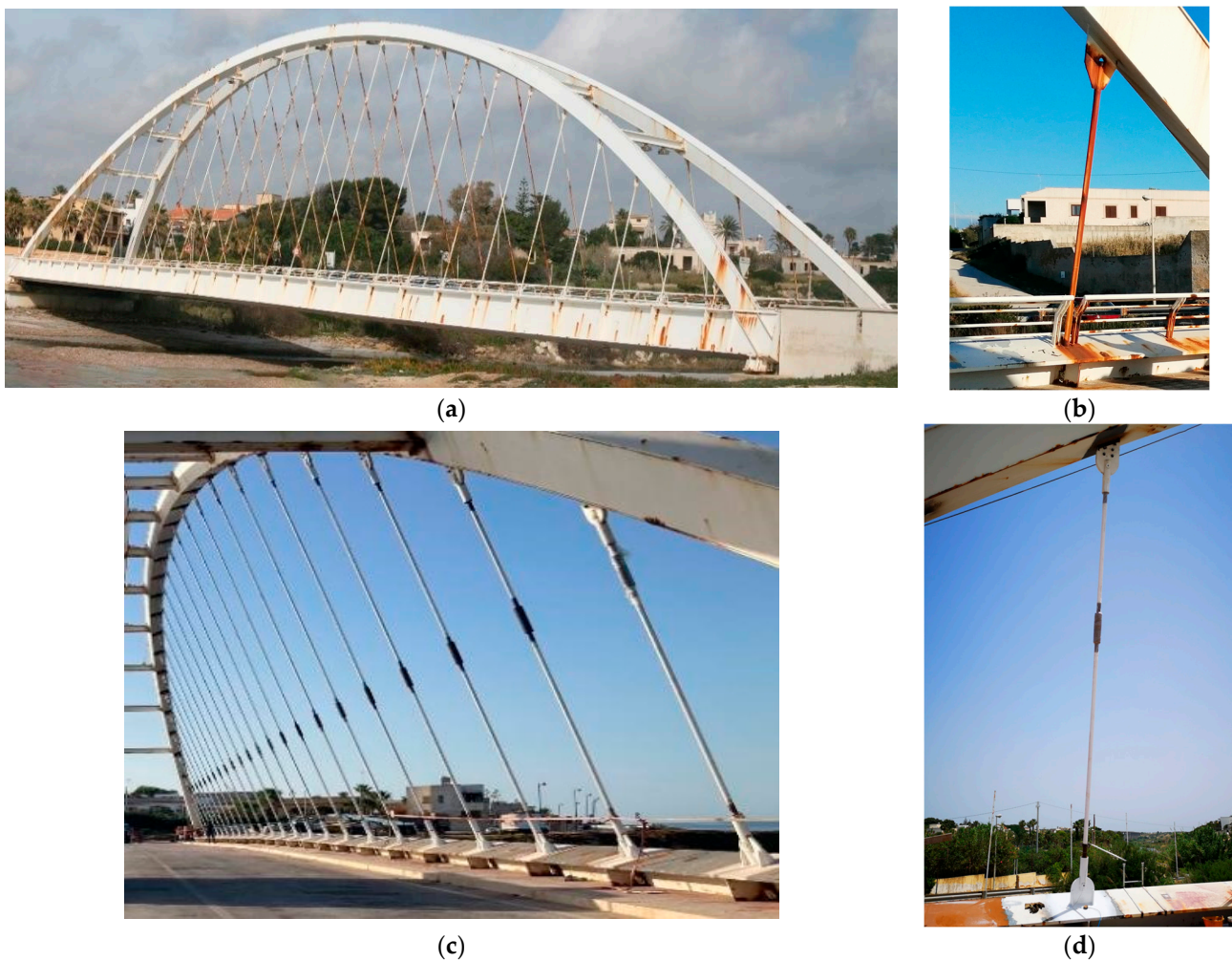
Figure 1. The case study bridge. (a) Original configuration; (b) original hanger with welded connections at the end; (c) new suspension system; (d) new hanger with end connections and intermediate tensioner.
