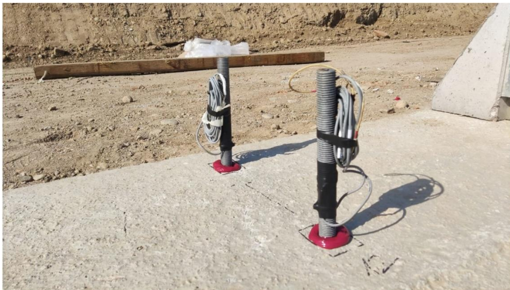
Fig. 4. Instrumented anchor bolts. Source: designs and photos are made by the Authors
