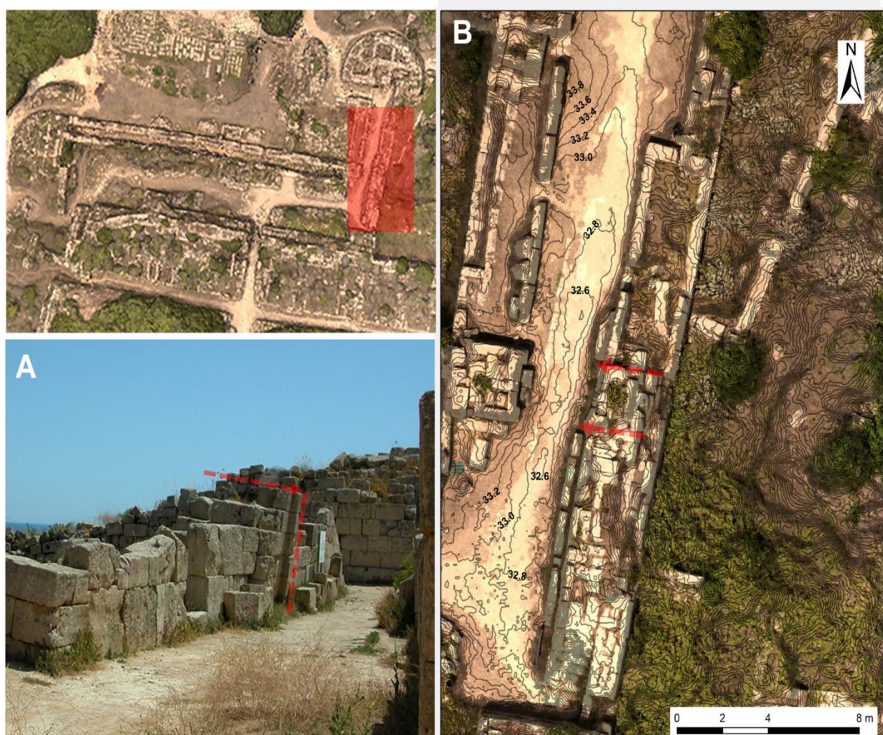
Figure 5: Gate XVIII sector. The frontwards movement of the inner defensive wall: A): the picture of an inner sector of the defensive wall, the slipping movement in red; B) the Orthophoto combined with DSM shows the depression at the bottom of the wall.
