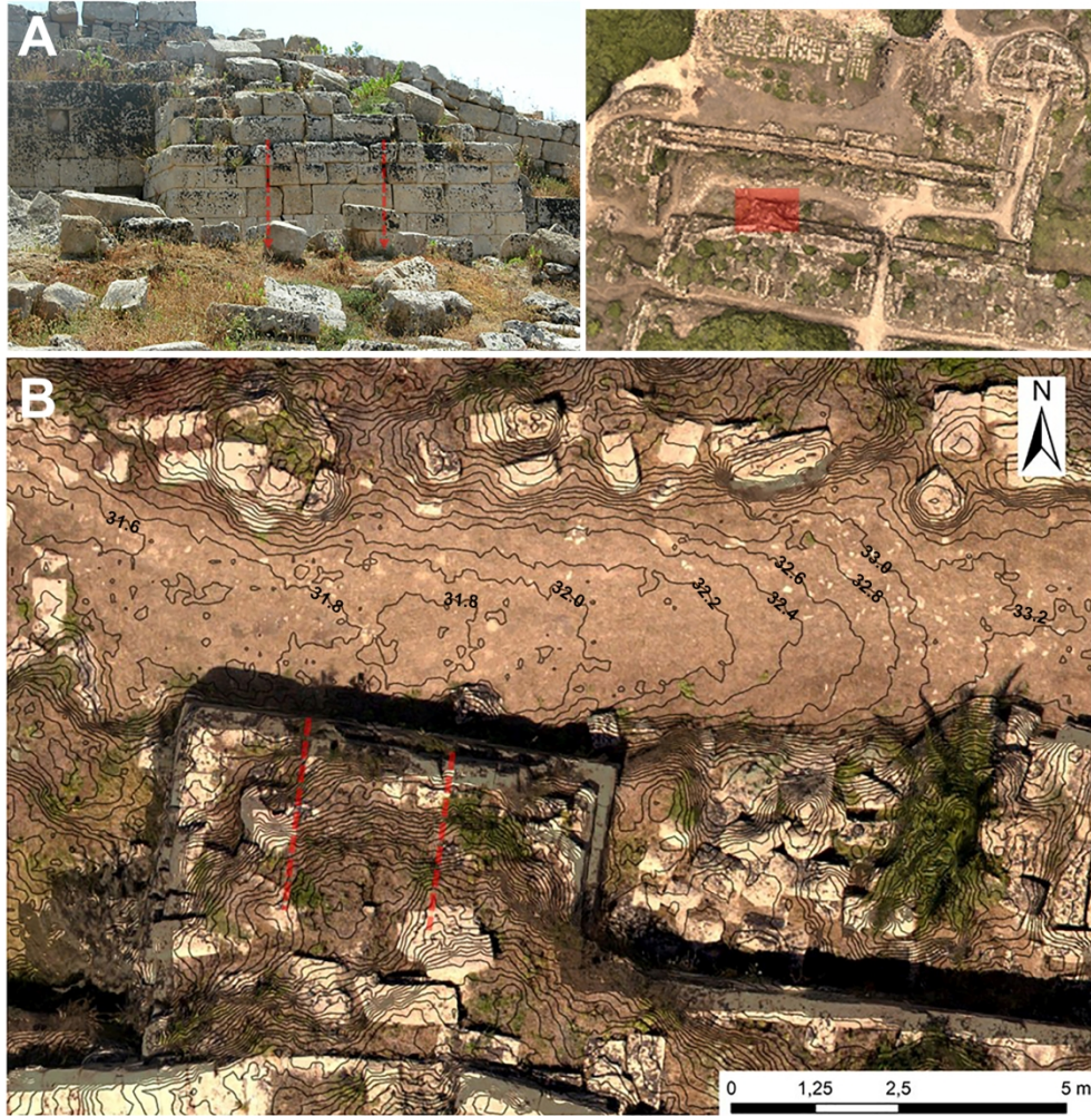
Figure 4. Northern fortifications: square tower along the external wall axis. The typical pattern cracking due to differential subsidence on defensive: A) the picture of a sector of the defensive wall, the main cracking system in red; B) the Orthophoto combined with DSM shows the depression at the bottom of the masonry.
