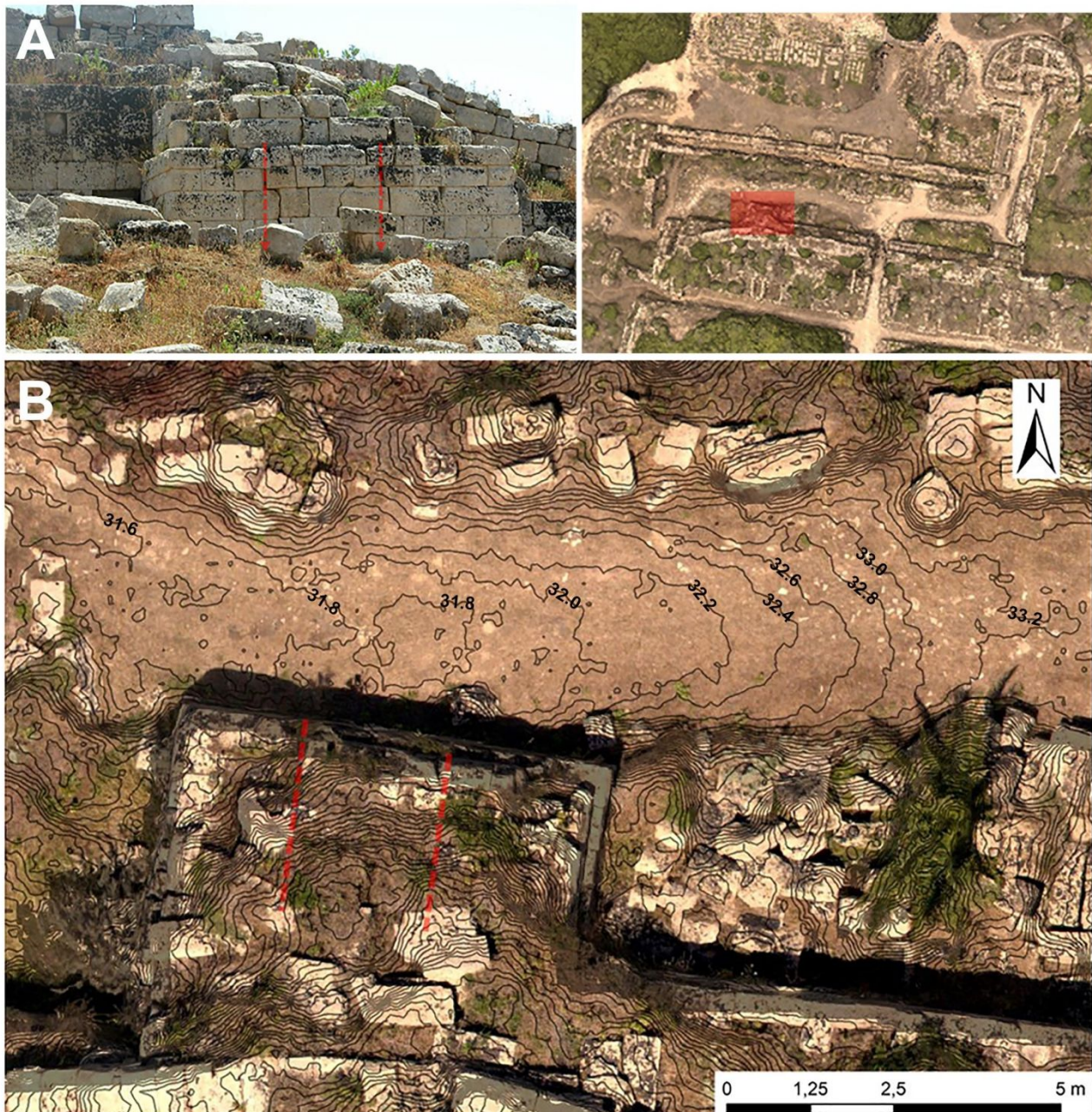
Figure 4. Northern fortifications: square tower along the external wall axis. The typical pattern cracking due to differential subsidence on defensive: A) the picture of a sector of the defensive wall, the main cracking system in red; B) the Orthophoto combined with DSM shows the depression at the bottom of the masonry.
