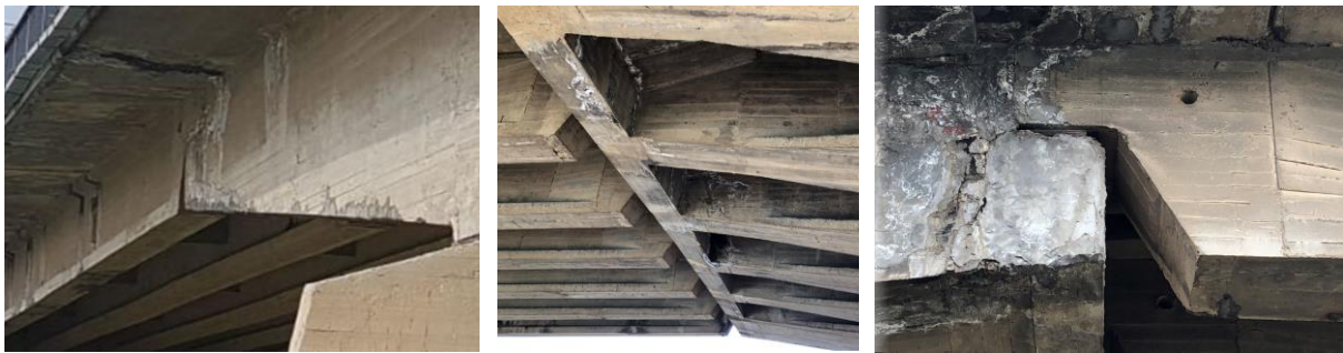
Figure 6. Deterioration of the Gerber saddles.
