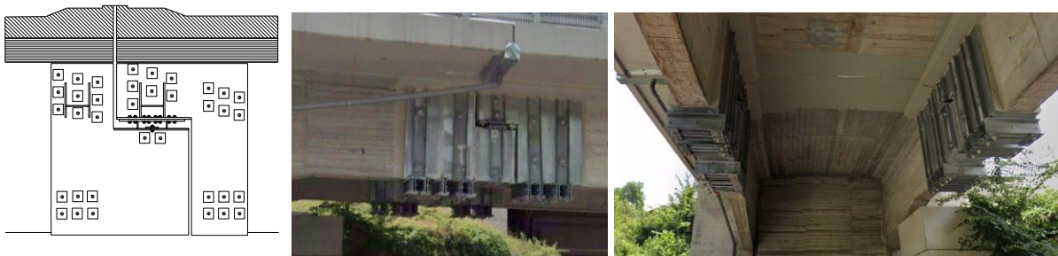
Figure 18. Steel plating of Gerber saddles of Sabbione and Generale Franco Romano viaducts (Italy) [19]
