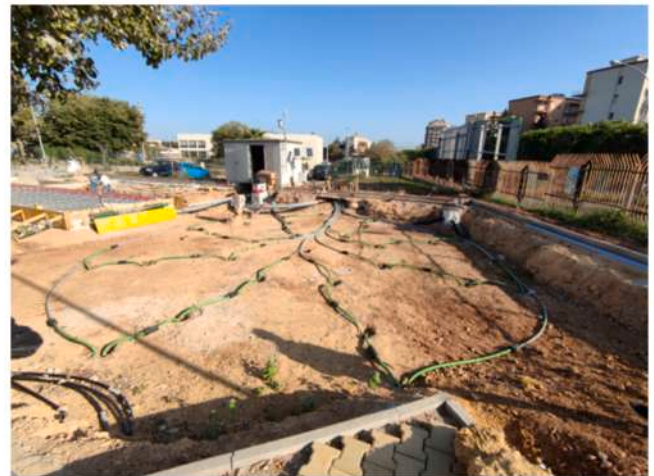
Fig. 11. Installation phase of the SMARTEP BTES System at the University of Palermo.
