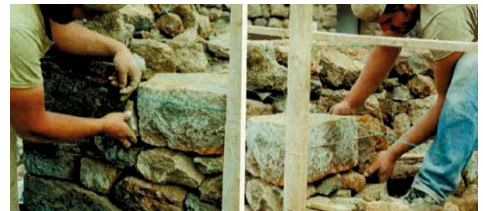
Fig. 5. Wooden scaffolding and line for the construction of a dry stone wall (Source: Progetto Medstone, 2002)
