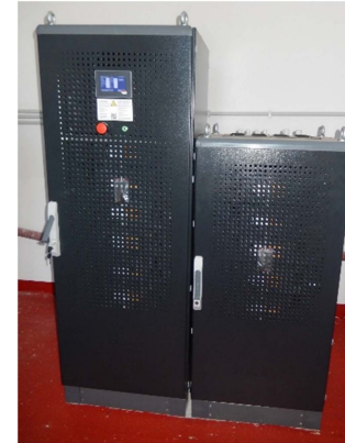
FIGURE 14. Battery of 20 kWh ESS.
