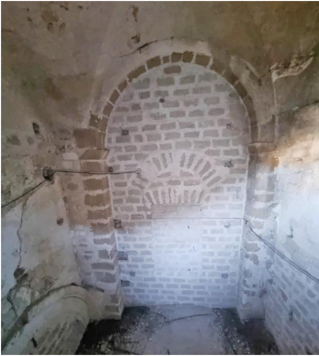
Fig. 10: View of the wall separating the presumed dismissed transept from the tribune: walled-up arch and traces of the blind window.
