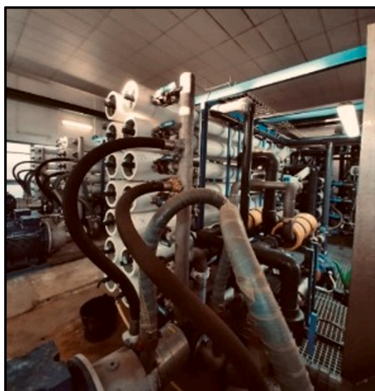
Fig. 1. Sataria SWRO Plant, Pantelleria (IT).
