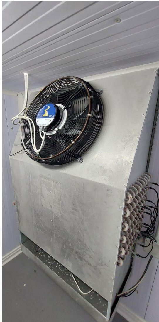
Figure 38 Finned-Tube Heat Exchanger (Evaporator)
