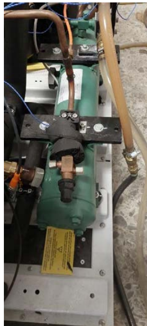
Figure 37 Water-Cooled Shell-and-Tube Heat Exchanger in Experimental Setup
