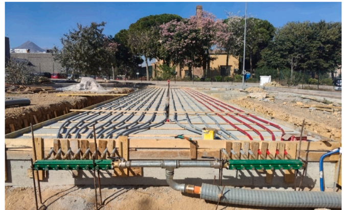
Fig. 3. Installation of the pipes of the SMARTEP RTC and connection with the manifolds.
