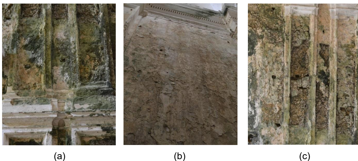
Figure 139. a) Biological colonization affecting the pillars; b) blistering of the plaster layer; c) Crumbling of the internal sandstone layers.
