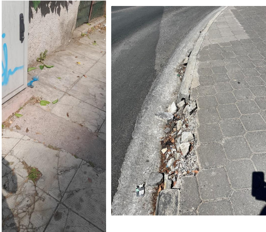
Figure 5–6. Utility Cut Patching (left) and edge cracking (right)
