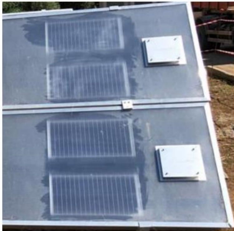
Figure 6.6 - Photovoltaic power supply for engine
