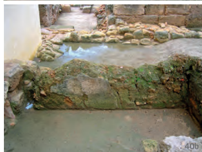
Fig. 40a, b: Marsala. San Gerolamo area. Residential building, Hellenistic-Roman period; the two sides of the same wall with an earthen upper wall (photo M. Schiera 2008). Evidence of lichen and the absence of floor drainage can be observed.
