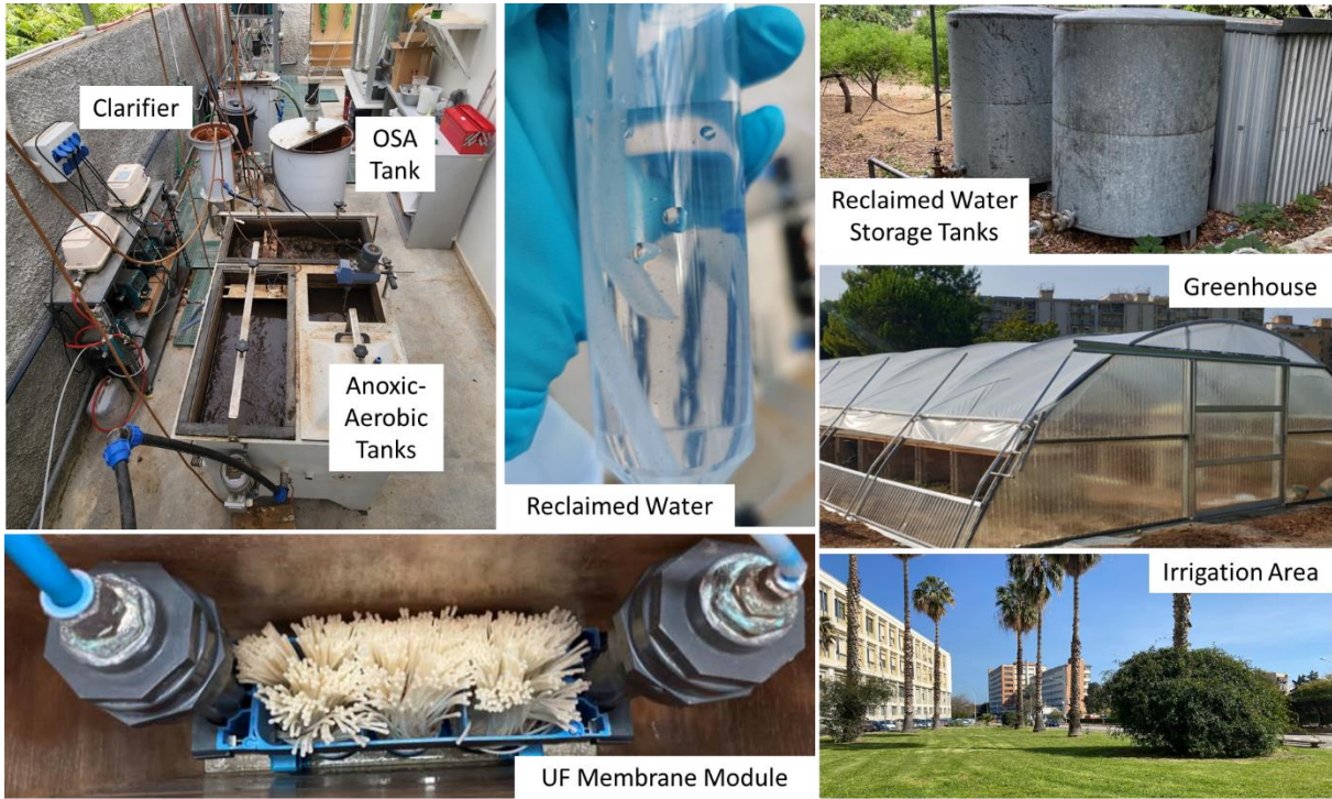
Figure 6. The pilot plant for wastewater treatment and water reuse system in Palermo University Campus
