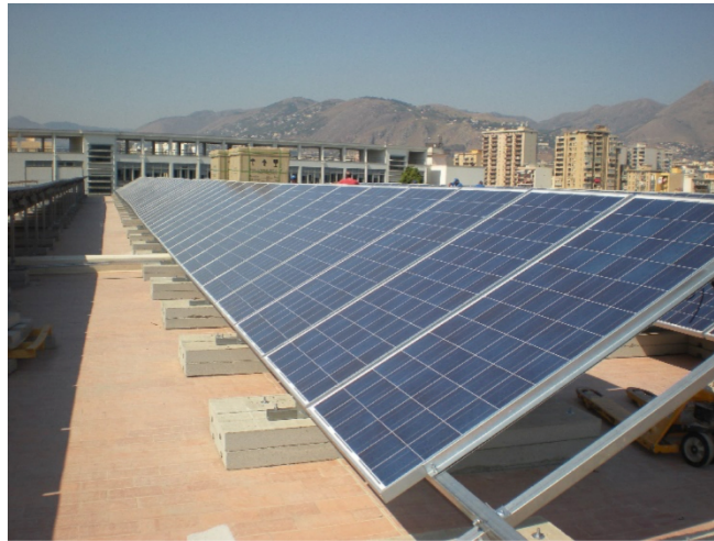
Figure 12.3. The large PV system on the coverage of a university building.
